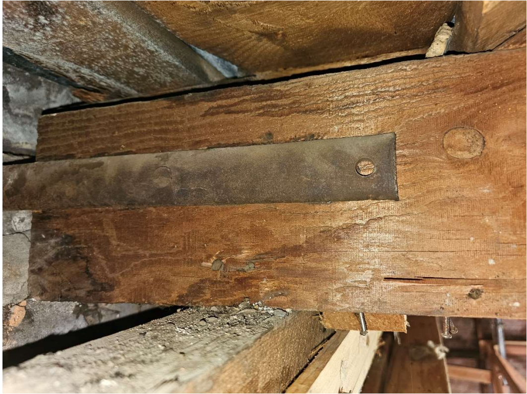
Photo #14: Roof truss wall anchor (Confidence Engine Company Hall)
