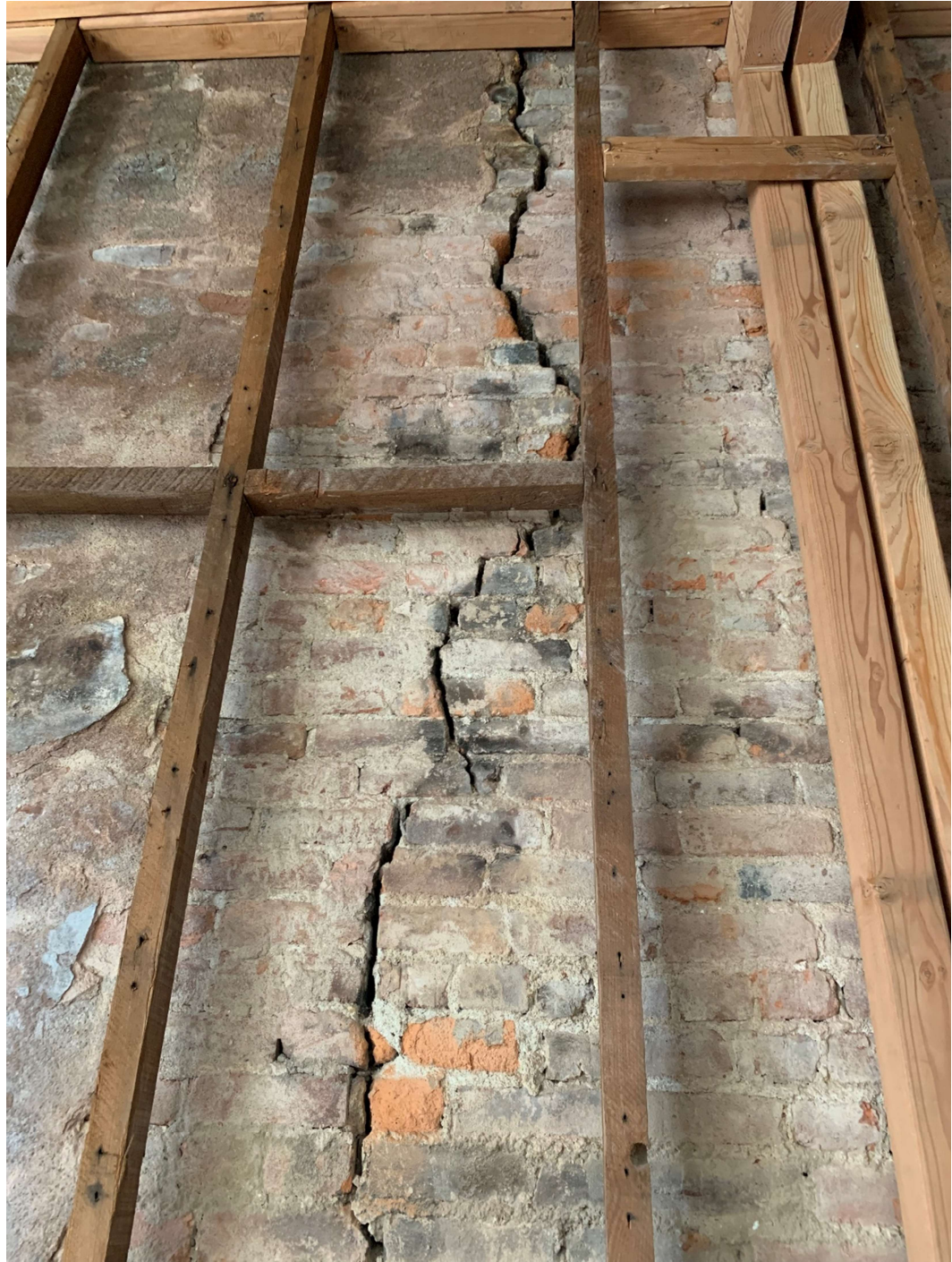
Photo #10: Crack in brick wall (West wall end)
