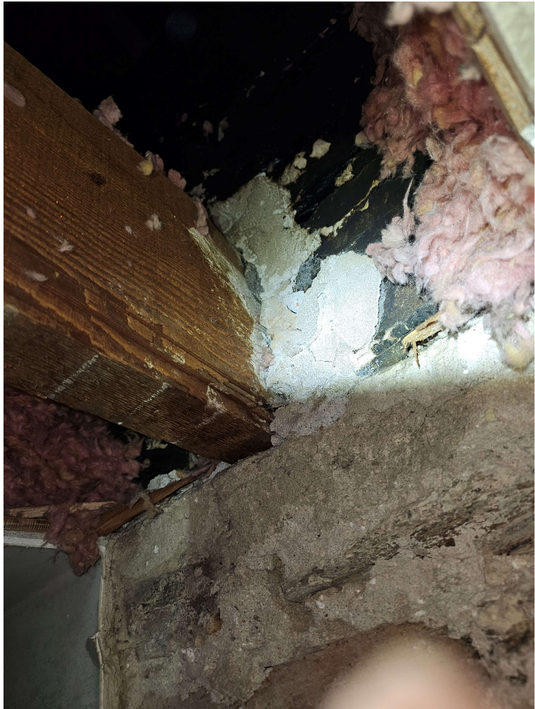
Photo #16: 2 nd Floor Interior Rock (below 2nd) to Brick (above 2nd) Transition
