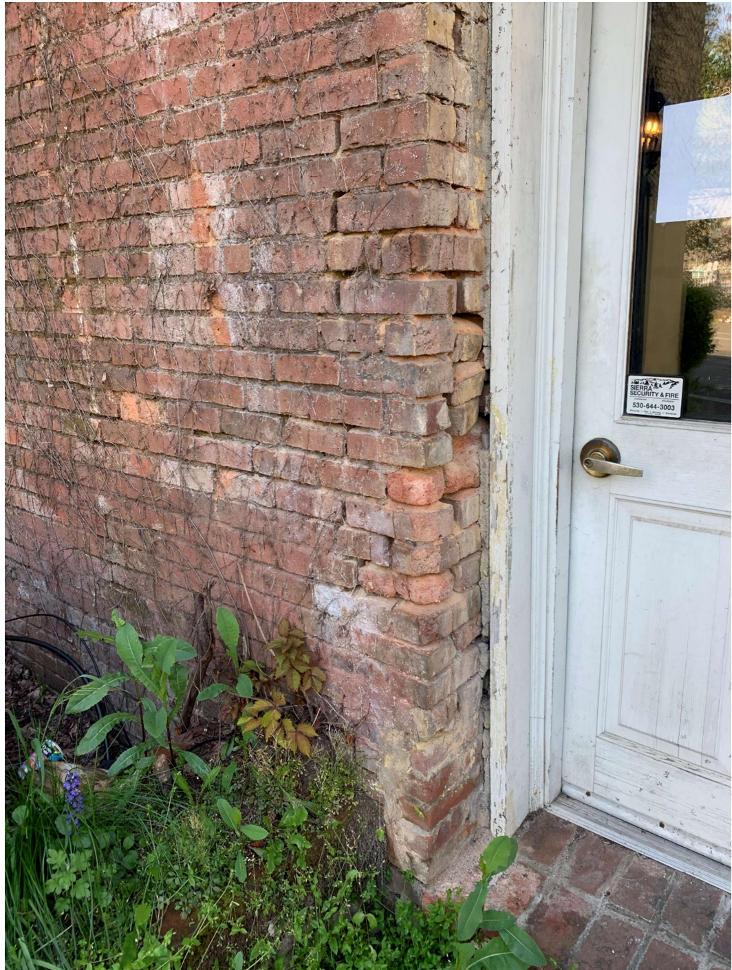
Photo #9: Brick damage near door jamb at Confidence Hall building
