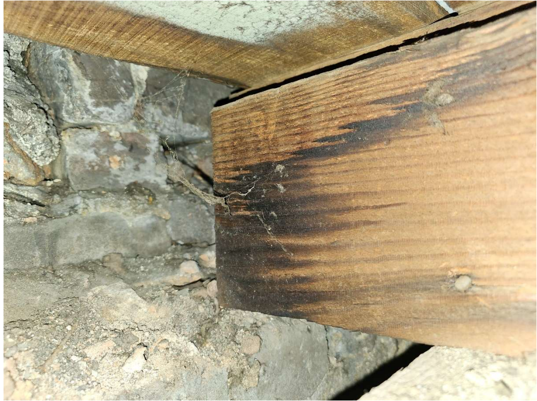
Photo #13: Company Hall Building Roof Trusses West wall support displacement
